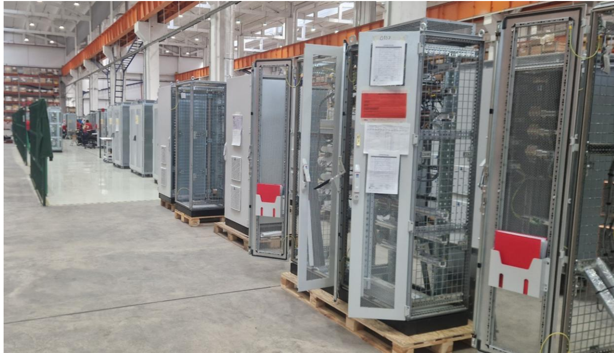
Korridor B HVDC control cabinets 7mEuro
